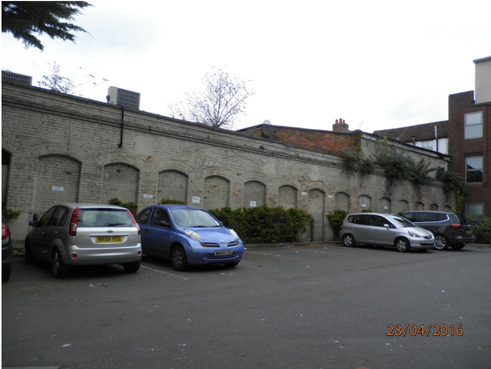
View of historic wall on southern boundary, from 118-128 London St. car park
