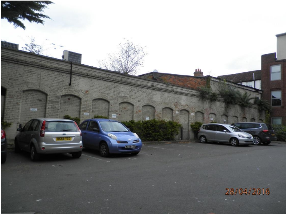
View of historic wall on southern boundary, from 118-128 London St. car park
